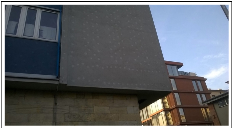
Figure 2. Façade of a building at Cracow TU after thermal upgrade with ETICS having a thick layer of thermal insulation. Drying on mechanical fasteners is faster than adjacent insulation that is still wet from morning condensation. Source: Photo courtesy of Tomasz Kisilewicz.
