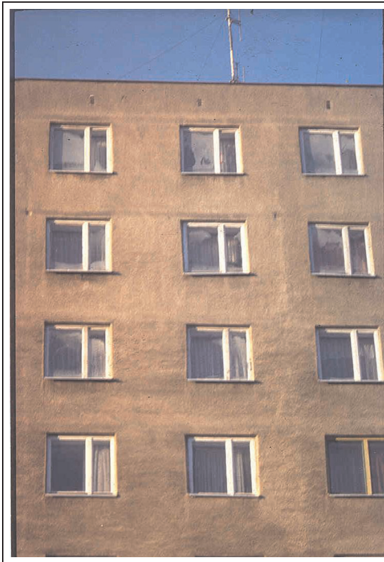
Figure 6. Tall building in cold climate in Europe, in winter. Stack effect caused air exfiltration demonstrated by frost visible on external glazing surface in double windows on the top floors, while those at the bottom of the building are clear. The connecting element for airflows here is a staircase.
